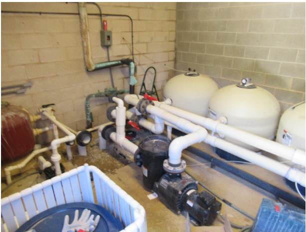
Filters and pumps overview
