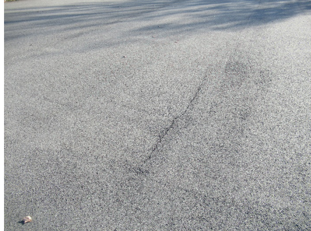
Crack at Dugout Terrace
