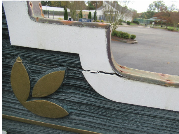
Rusted fasteners and cracks
