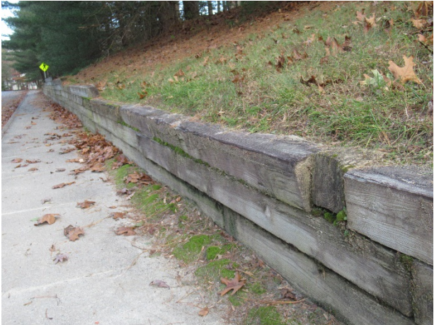
Timber retaining wall overview – Note: displacement and organic growth
