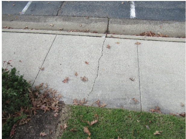
Concrete sidewalk crack
