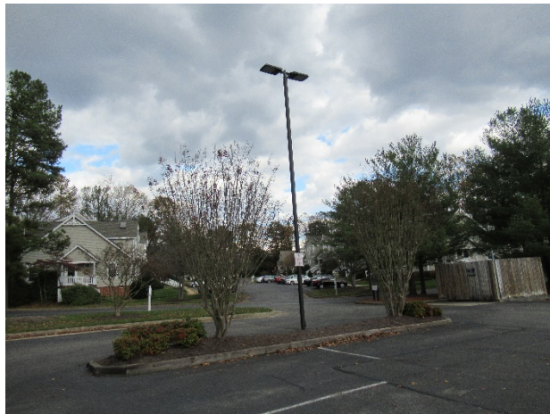
Parking lot light pole and fixture overview
