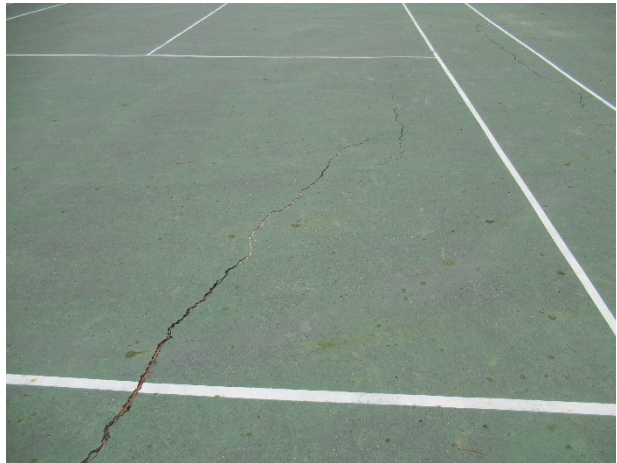
Crack at clubhouse
