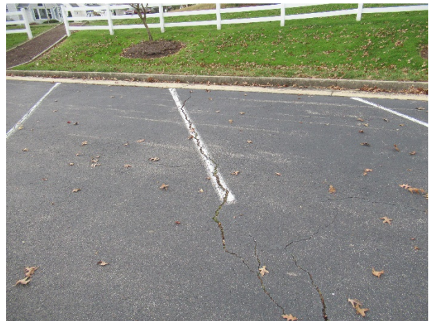
Asphalt pavement crack
