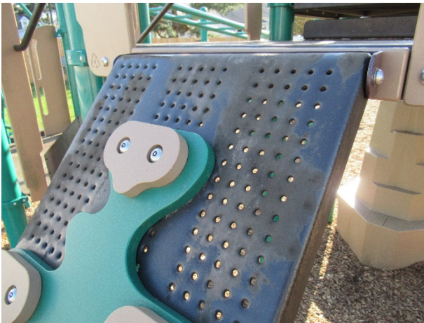
Wear at Dugout Terrace
