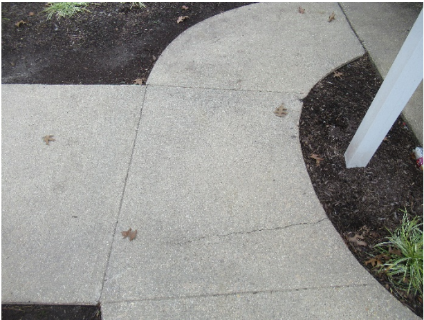
Concrete sidewalk crack
