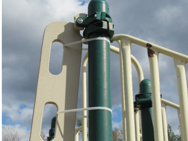
Loose equipment at clubhouse
