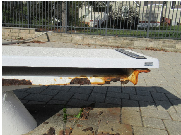
Diving board rust
