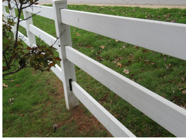
Vinyl fence displacement
