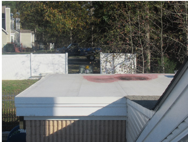
Thermoplastic roof overview – Note: standing water
