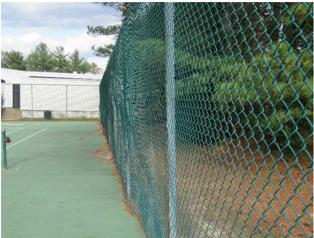
Clubhouse fence overview – Note: warping
