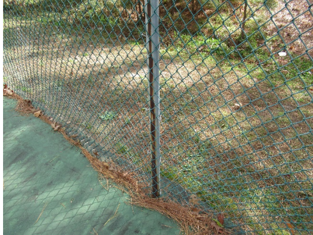
Finish deterioration at the clubhouse
