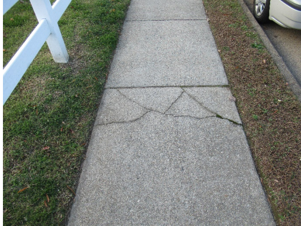
Concrete sidewalk cracks
