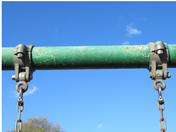
Rust and finish deterioration at Dugout Terrace
