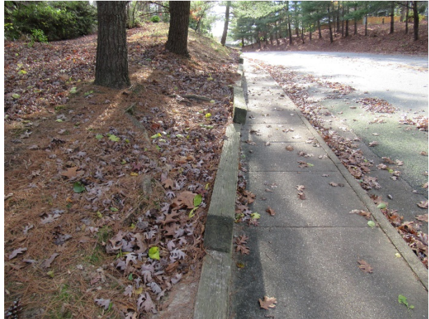
Timber retaining wall overview – Note: lean
