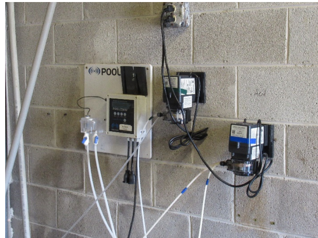
Automatic chlorinator overview
