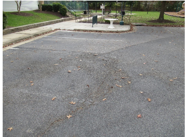
Asphalt pavement overview – Note: raveling
