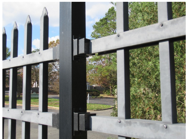
Replaced section and displacement
