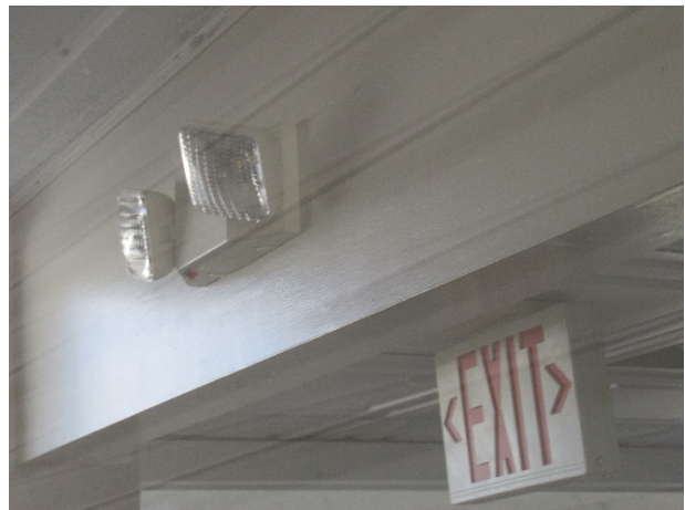
Emergency fixtures overview
