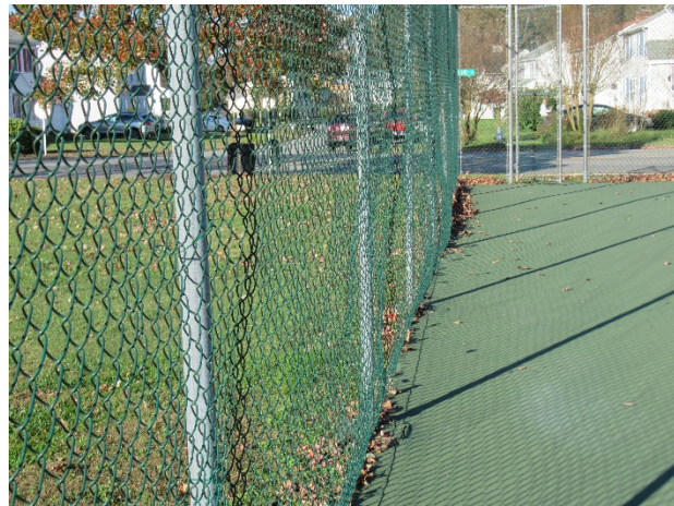
Dugout Terrace fence overview – Note: warping
