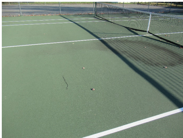
Crack and staining at Dugout Terrace
